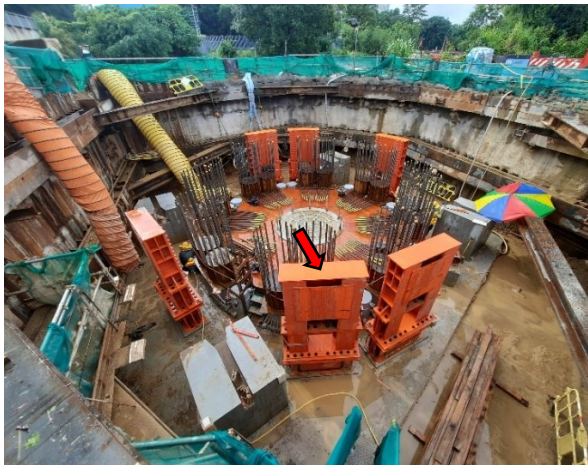
Figure 4.13 - Temporary supports installed on lower turntable prior to the casting of upper turntable
