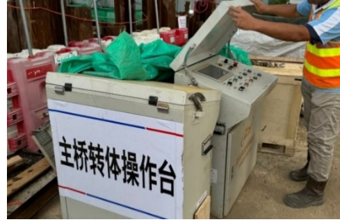
Figure 4.38 - Control station for hydraulic strand jacks
